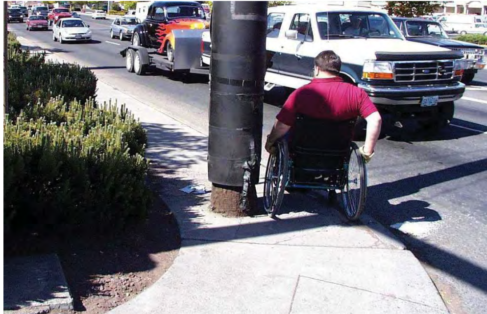
Obstructions can make passage difficult or impossible for wheelchair users. (Credit: Michael Ronkin)
